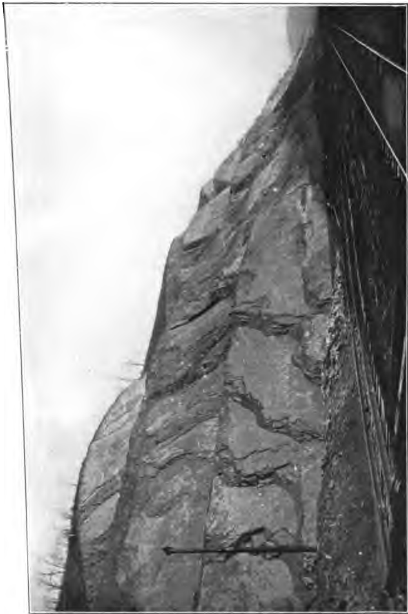
PLATE XXXVII.—View showing Flaggy Character of Catskill Sandstone in Doe Gully Cut of Baltimore and Ohio Railroad.
